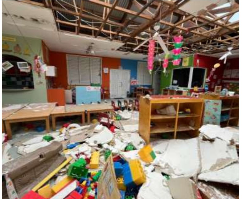
Owia Government School, Northwindward Saint Vincent and the Grenadines damaged by Hurricane Beryl. Photo: UN RCO Barbados and the Eastern Caribbean.
